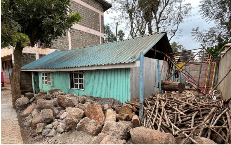
Current Kitchen & dining room. A 3-story addition will replace this structure (1st floor – Kitchen; 2 nd floor – dining room; and 3 rd floor – classrooms)
